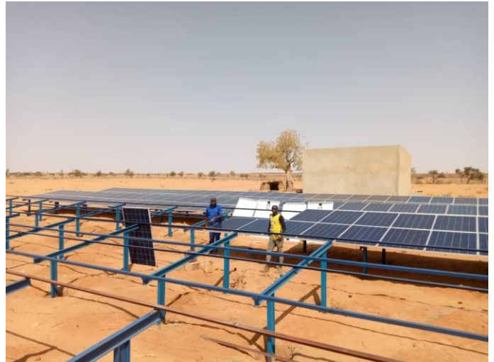
A new solar installation made by Solafrique
