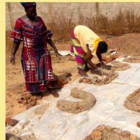
Workshop for building wood solar ovens for the woman members of Notre Soleil
