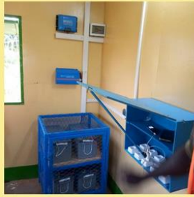
A mobile phone charging station in a solar kiosk's kitchen area
