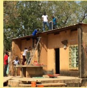
Solar installation in the Catholic center of Kouentou, installed by Solafrique (2016)
